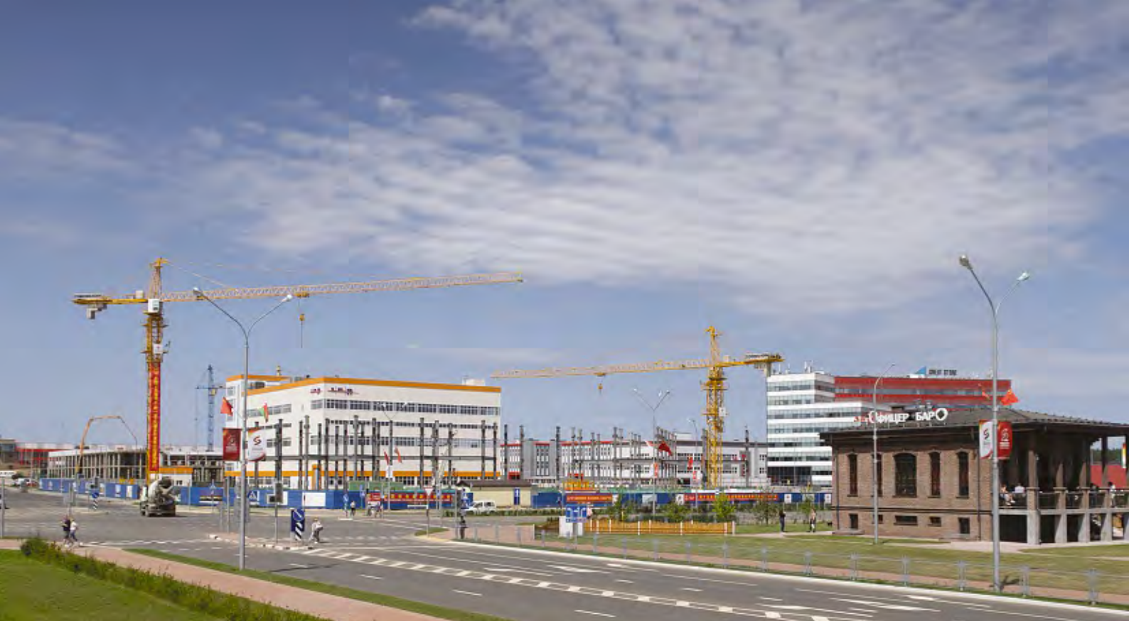
BRI cornerstone: Great Stone Industrial Park is 25 kilometres from Minsk and has been in development since 2010
